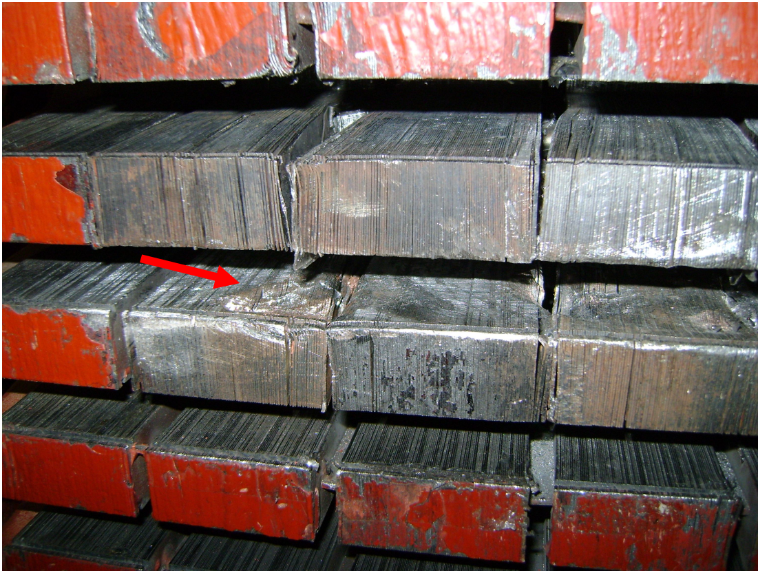
2. Core fault seen in slot 14.
