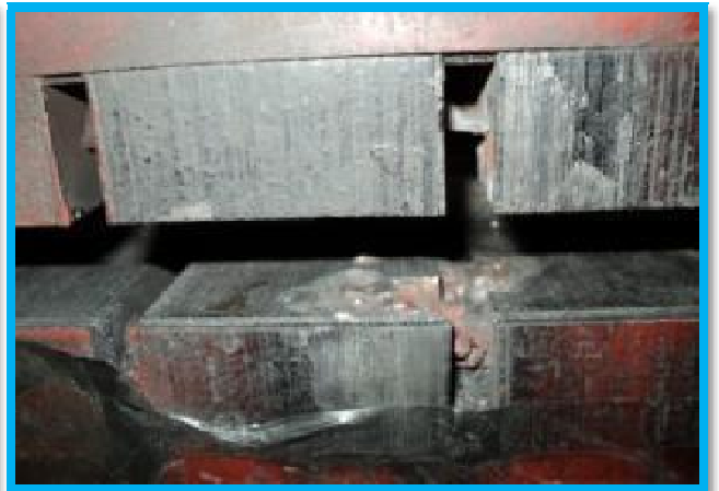
Photograph 4: Core Damage (Lower side)
