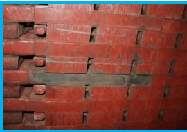
Photograph 1: Missing End Wedge
