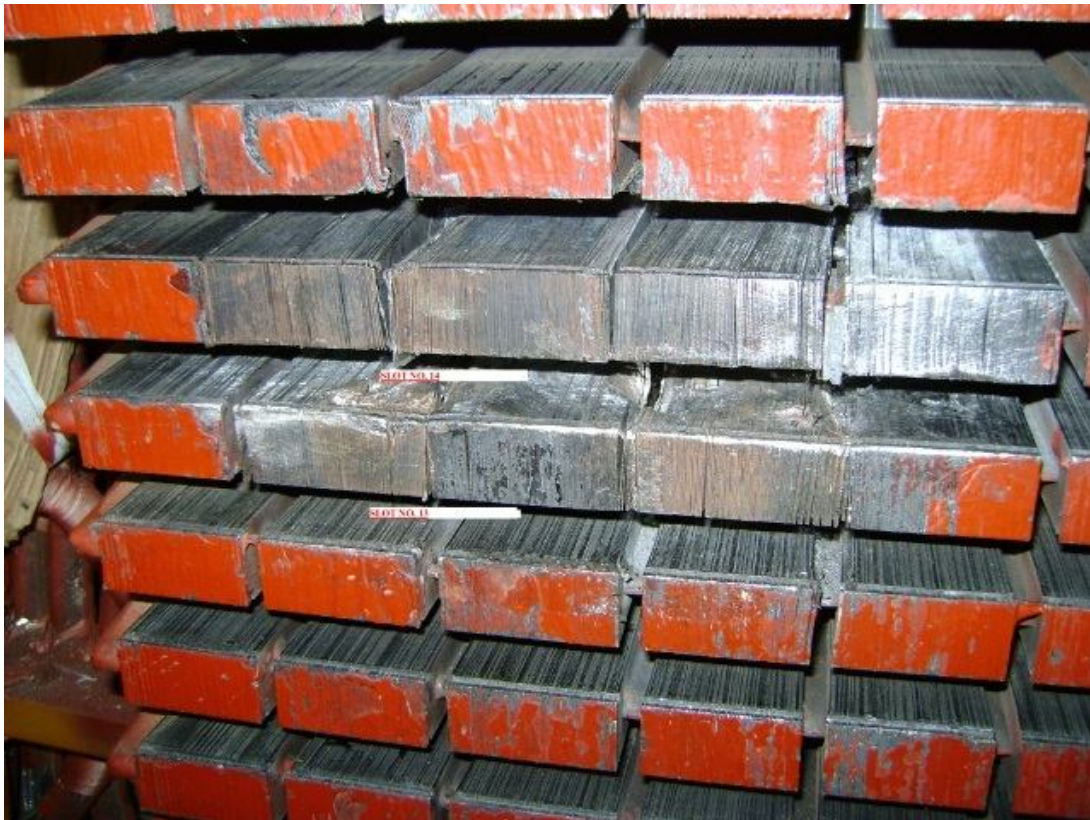
1. Core fault seen in slot no. 14
