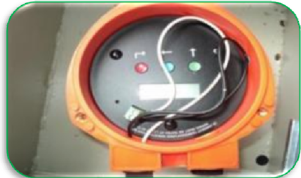
Control panel for device at Control Room
