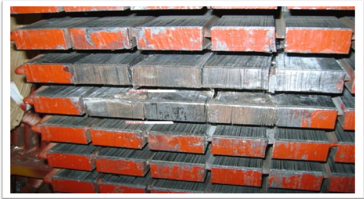
Photograph 14: Core Faults seen in Slot no. 14
