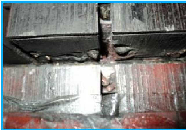
Photograph 3: Core Damage (Upper side)
