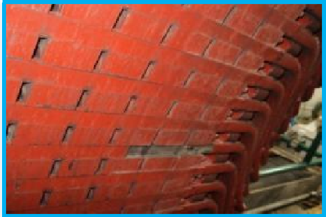
Photograph 6: Missing End Wedge
