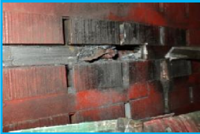
Photograph 5: Pitted Stator Core Segment
