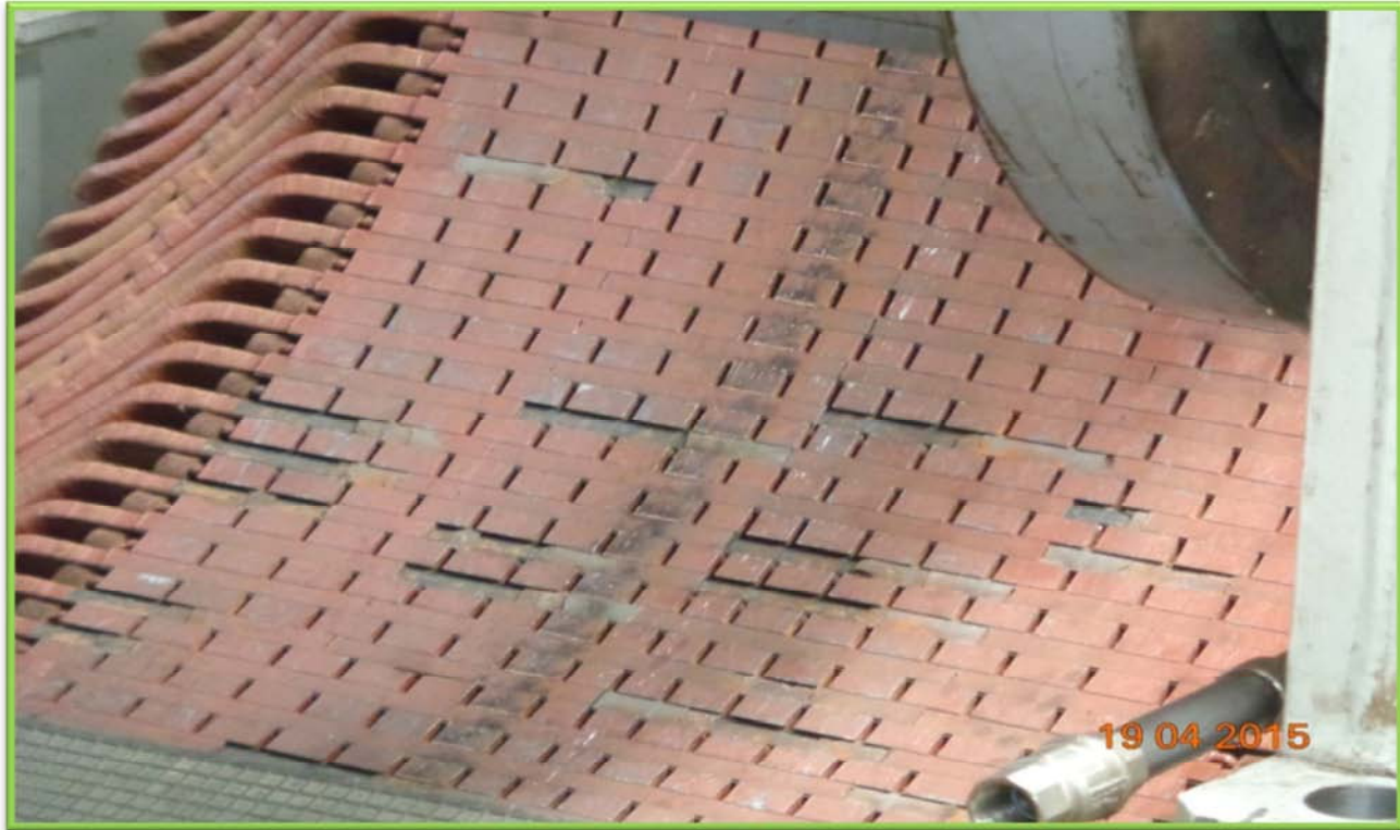
Photograph showing Scratches observed on stator of unit 2
