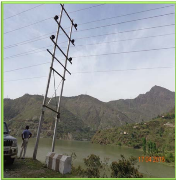
Tilted pole due to slide of foundation
