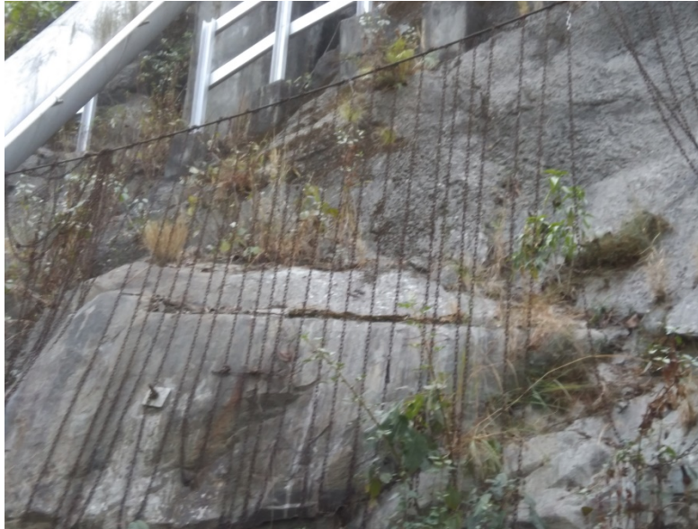
Steel Chains provided u/s of Power House
