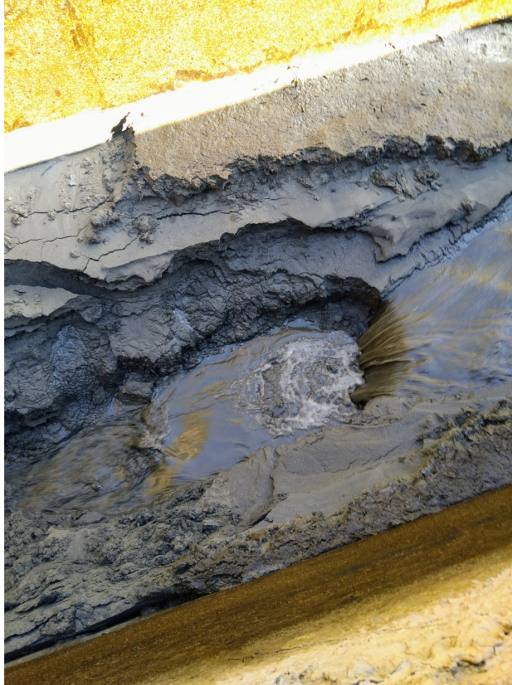
Silt Deposition in Desilting Chamber
