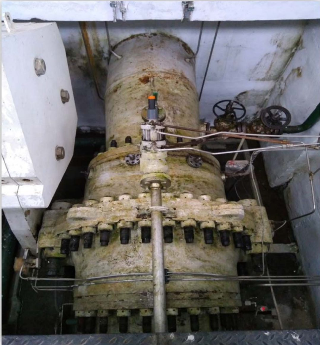
Rusting on Penstock/MIV during Site Visit
